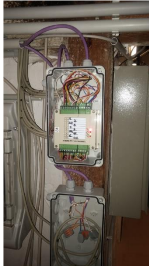
Fig. 13 Installed 3T-Pt10 Pt 100 transmitter
