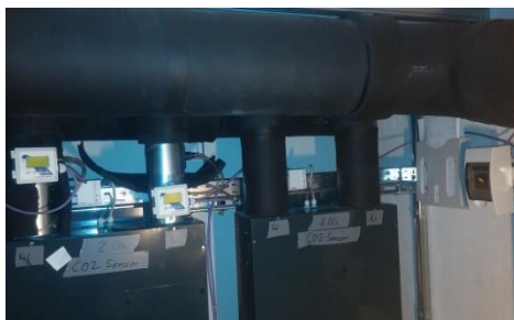
Fig. 10 CO 2 sensors for heat exchanger 2G
