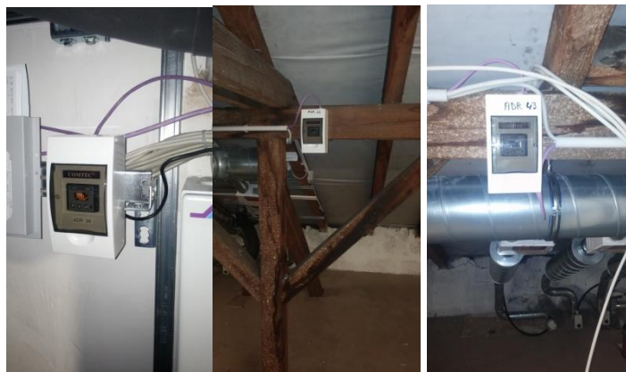
Fig. 9 From left to right Power network meter: heat exchanger EG Site 2, ventilator 3 right Site 1, ventilator EG right Site 1
