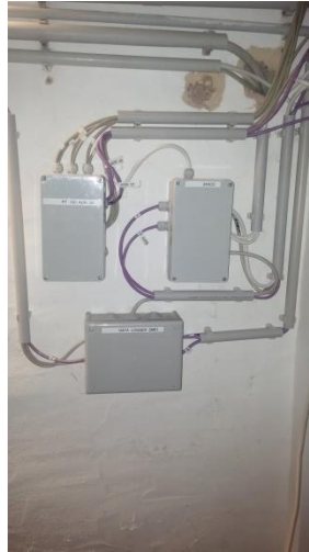
Fig. 20 SM61 enclosure montage in Site 2
