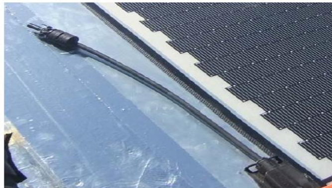
Figure 6. Photo of an electric connector to the PV module.
